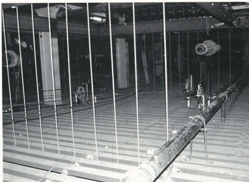
The grid as it is today. Chain hoists still have their uses.
